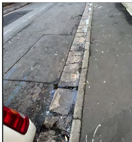
Condition 5 – Very poor
