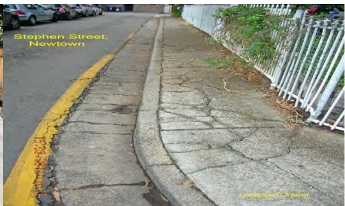
Condition 5 – Very poor
