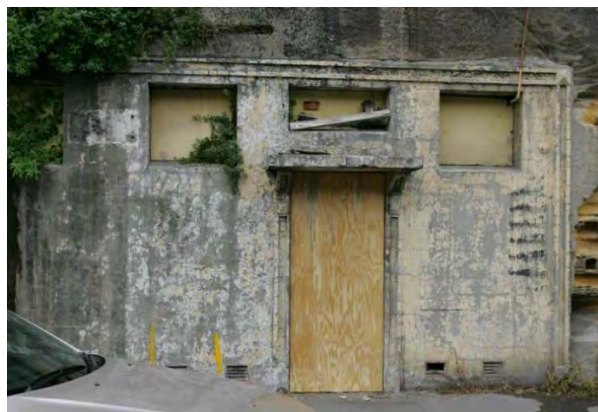
Condition 5 (very poor)
