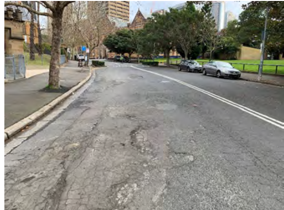
Condition 5 – Very poor
